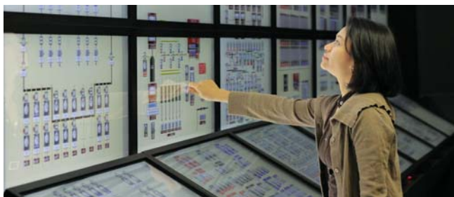
The EC6 Control Room features touch-enabled video display units.
