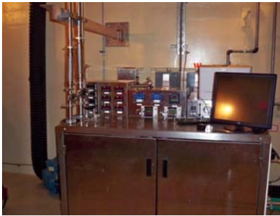
E1000LT VDS Installed in the Spent Fuel Pool Building.
